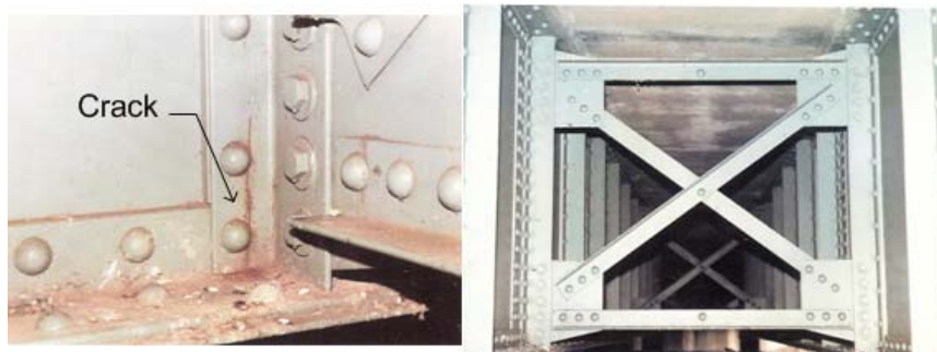
Figure 5 Fatigue cracking in the riveted connection of cross-bracing elements.
